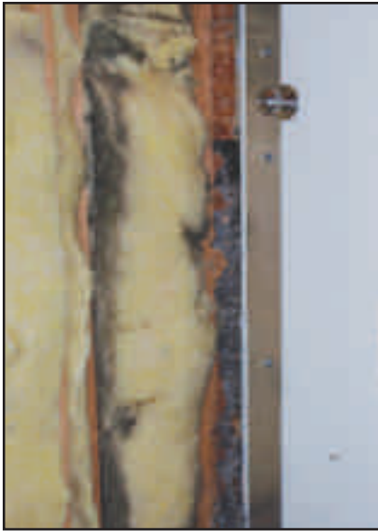
Signs of interior mould.
